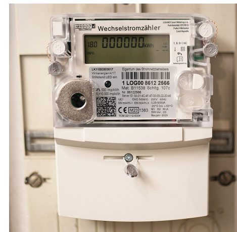
A household electricity meter counts the energy used, in kilowatt-hours (kWh) — the number it shows is what you pay for
