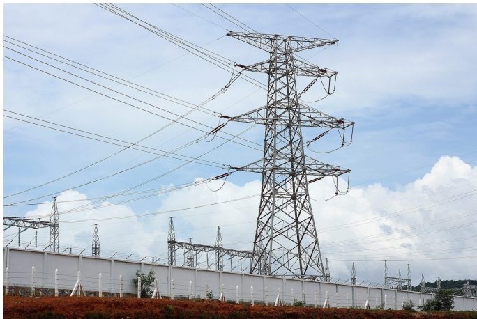
High-voltage power lines: electrical power is transmitted as high voltage so current (and I^2 R loss) stays low
