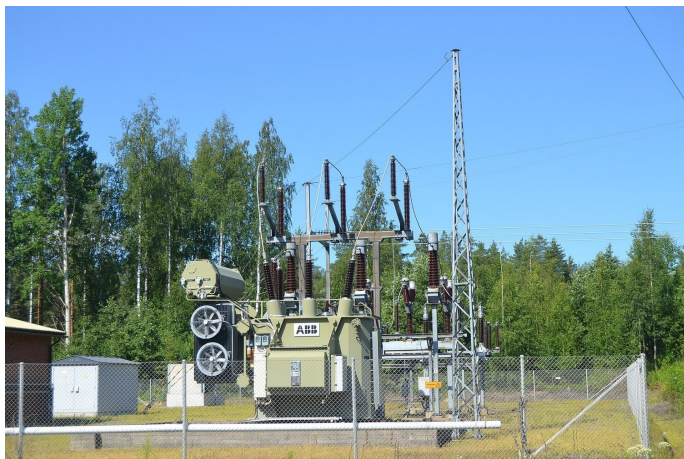
A substation transformer: changing magnetic flux in coils induces the voltages that power the grid
