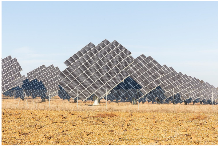
Solar panels in Spain
