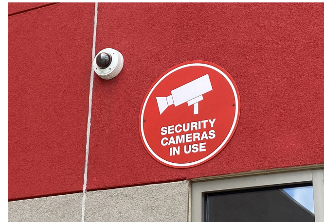
A dome security camera: physical controls and monitoring protect spaces as well as networks
