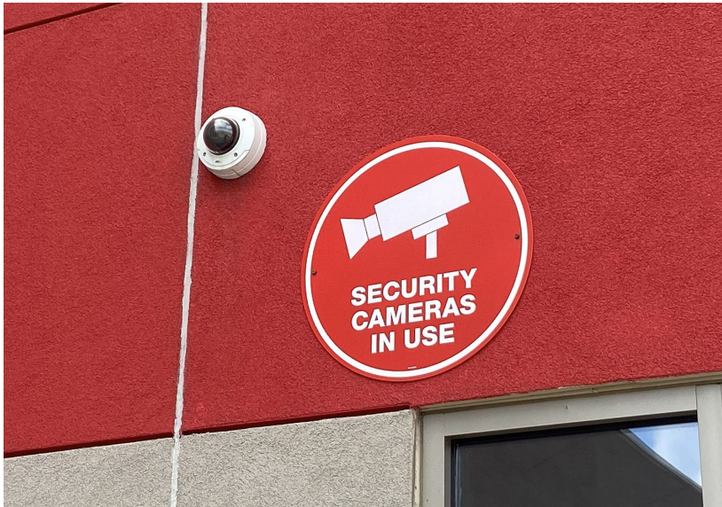
A dome security camera: physical controls and monitoring protect spaces as well as networks
