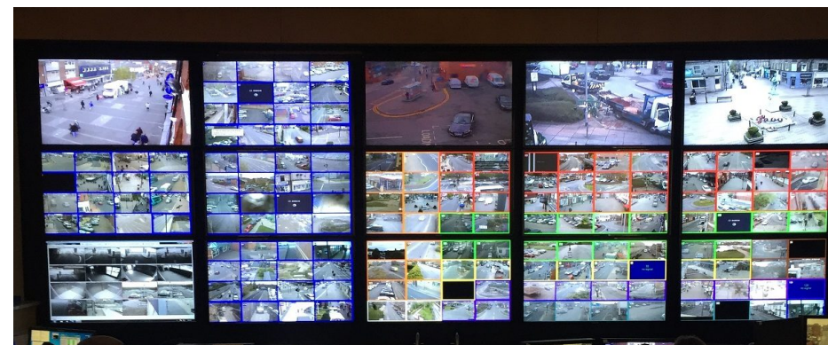
A CCTV control room: surveillance systems trade safety gains against privacy concerns
