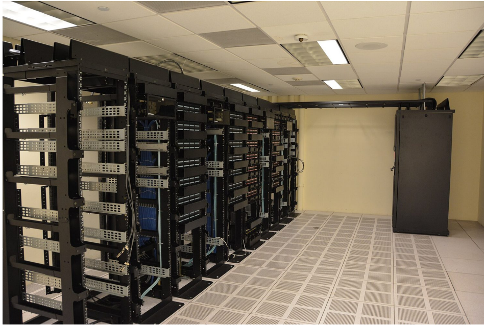
Large modern databases are stored on servers in data centres
